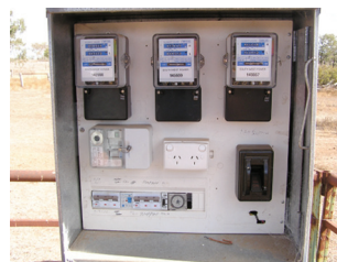
Figure 2: Power authority meters at end of overhead service line
