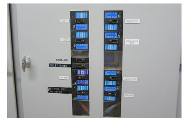
Figure 3: Typical distribution main board
